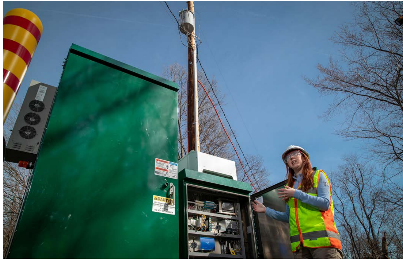
Nicole Lacouve, support engineer for PPL Electric, explains how a battery storage unit keeps customers in power and regulates voltage fluctuations on a power line.
