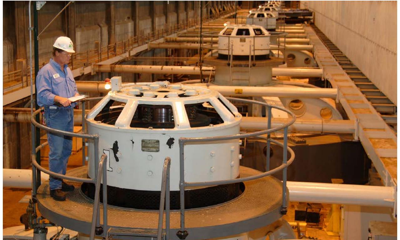
The Ohio Falls hydroelectric plant was recently upgraded, increasing the amount of clean energy generated by 25 percent.
