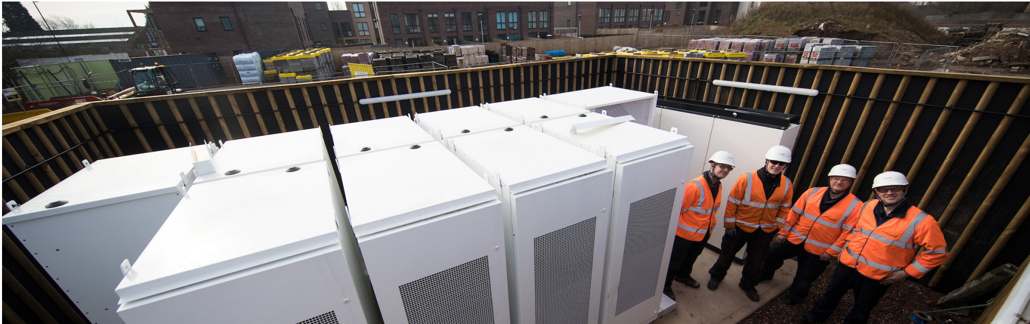
The battery system stores excess electricity generated by homes in this groundbreaking community energy project in Nottingham.
