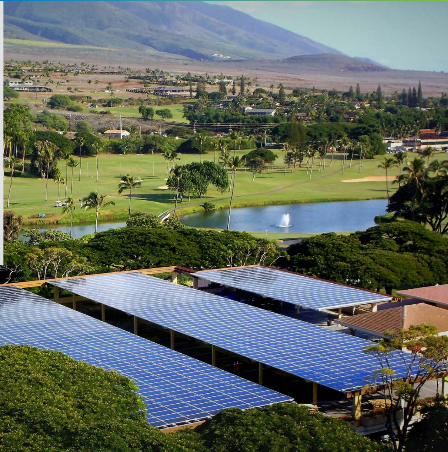
The Whalers Village solar project in Lahaina, Hawaii, is among the 200 solar generation systems installed by Safari Energy.
