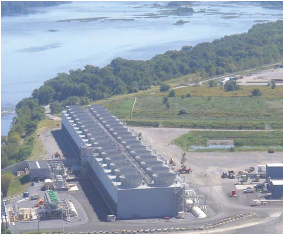
Tower will cool a half-million gallons of water every minute.
