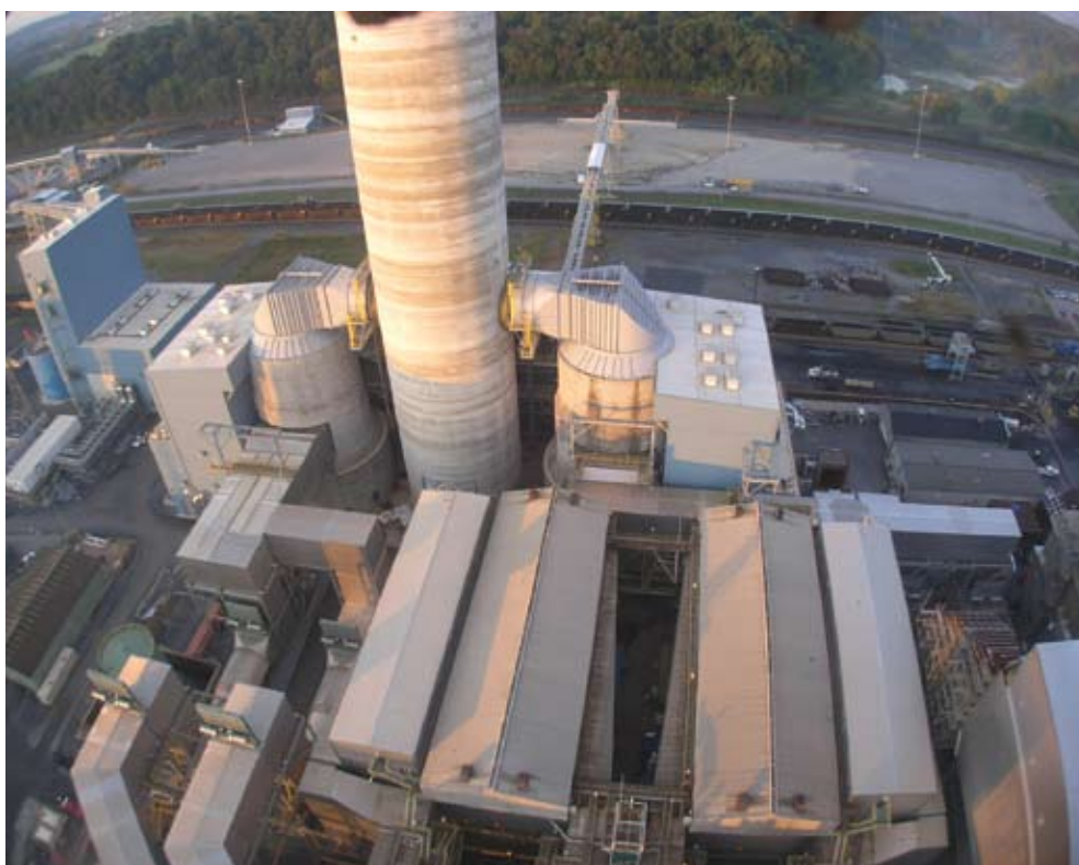
Unit 1 and 2 scrubbers will go into service later this fall.
