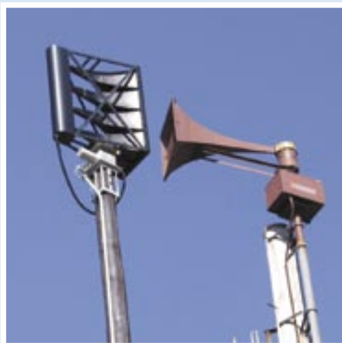
The new sirens (left) will rotate on their poles to ensure full coverage. The old sirens (right) will be removed after the new system is installed.
