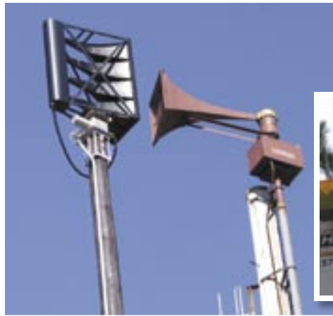
Most of the new sirens, pictured on the left next to an older siren, are installed.
