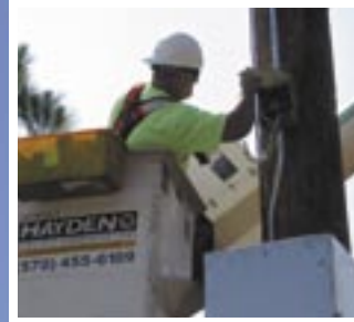
A worker installs the electrical connections to one of the new sirens.
