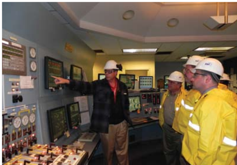
Montour plant manager Michael Munroe explains the information on a Control Room monitor during state Rep. Kurt Masser's visit to the plant.
