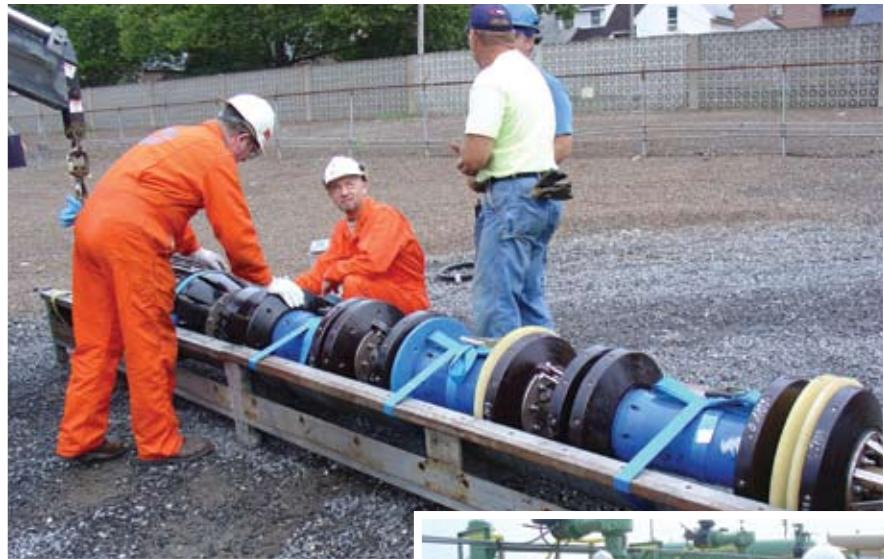
Workers prepare to insert a pig into the PPL Interstate Energy pipeline at Marcus Hook, Pa. The sophisticated monitoring device checks the entire 84-mile pipeline for corrosion.
