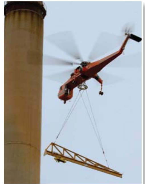
A helicopter performs an aerial ballet, gently positioning a crane atop the Unit 3 boiler.
