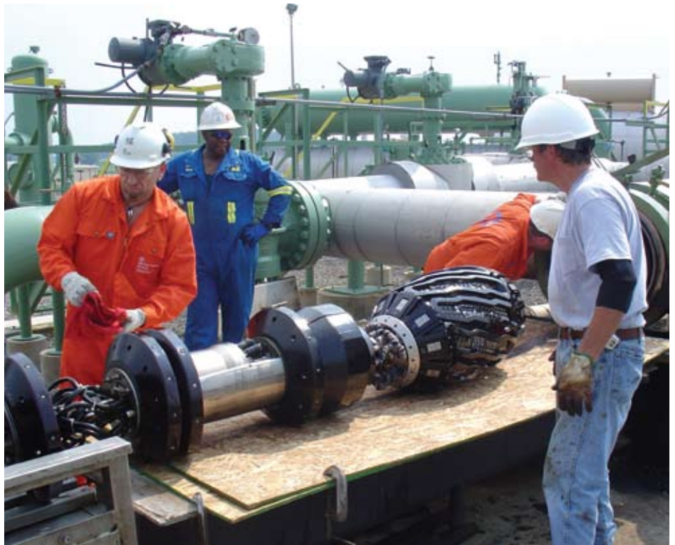
PPL Interstate Energy Company uses a pipeline "pig," seen here, to inspect its pipelines for damage .
