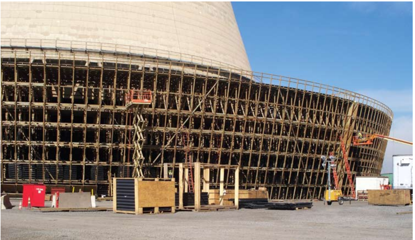
The new wooden structure encircling the base of the Unit 1 takes shape.
