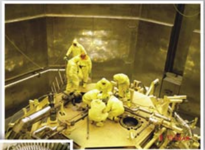
Above, crews prepare to open the reactor lid so they can replace more than 280 uranium fuel bundles.
