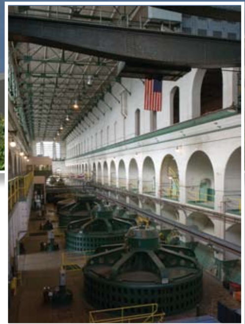
Interior view of Holtwood powerhouse.
