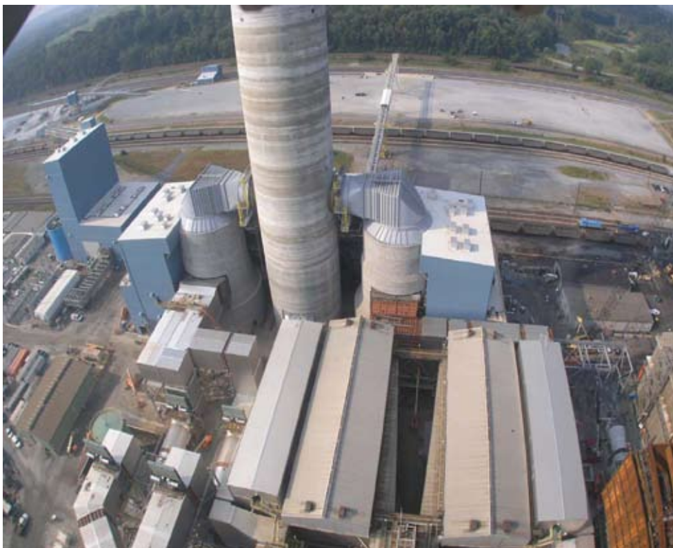
Duct work is now connected to either side of the new chimney stack as part of the scrubber project.
