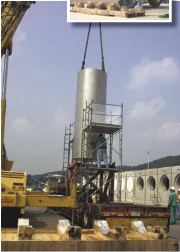
Workers lift one of the new dry fuel storage canisters onto a truck to take it into the plant to be filled.
