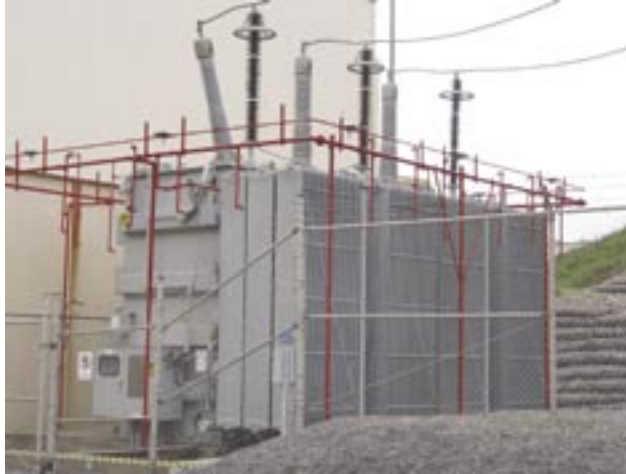
This transformer was replaced in October. Electricity demand in the United States has doubled since 1975. Nuclear energy provides more than 30 percent of the electricity produced in Pennsylvania and about 20 percent nationwide.
